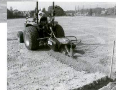
Work in progress in 2005 at Tunbridge Wells. The club were made a £6,000 grant towards the lifting and re-laying of three courts as well as installing an automatic watering system. It is only with the help of legacies made to the CA that grants such as these can be made.
