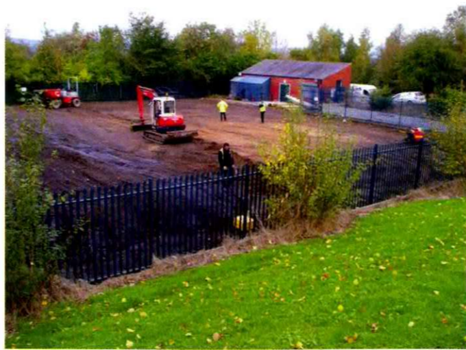
The old turf cleared and levelling can begin. Photo by Paul Rigge.
