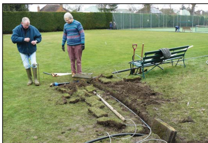
Mike Beaney and Tom Eddy start work on wiring up the solenoid control cable
