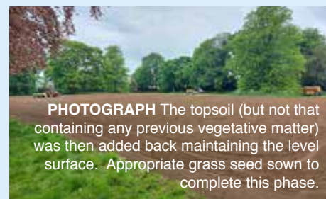
PHOTOGRAPH Removal of all the topsoil to get to the subsoil layer. All material moved was stored for re-use.
